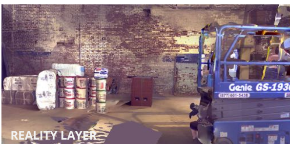
Construction site scan showing actual photo, point cloud, colored point cloud and Reality Layer photorealistic model
